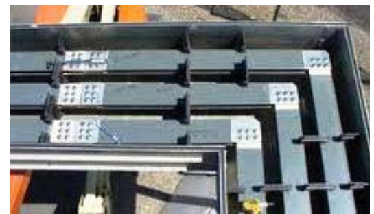
SCM monitors Switchgear, Cables and Bus Duct
